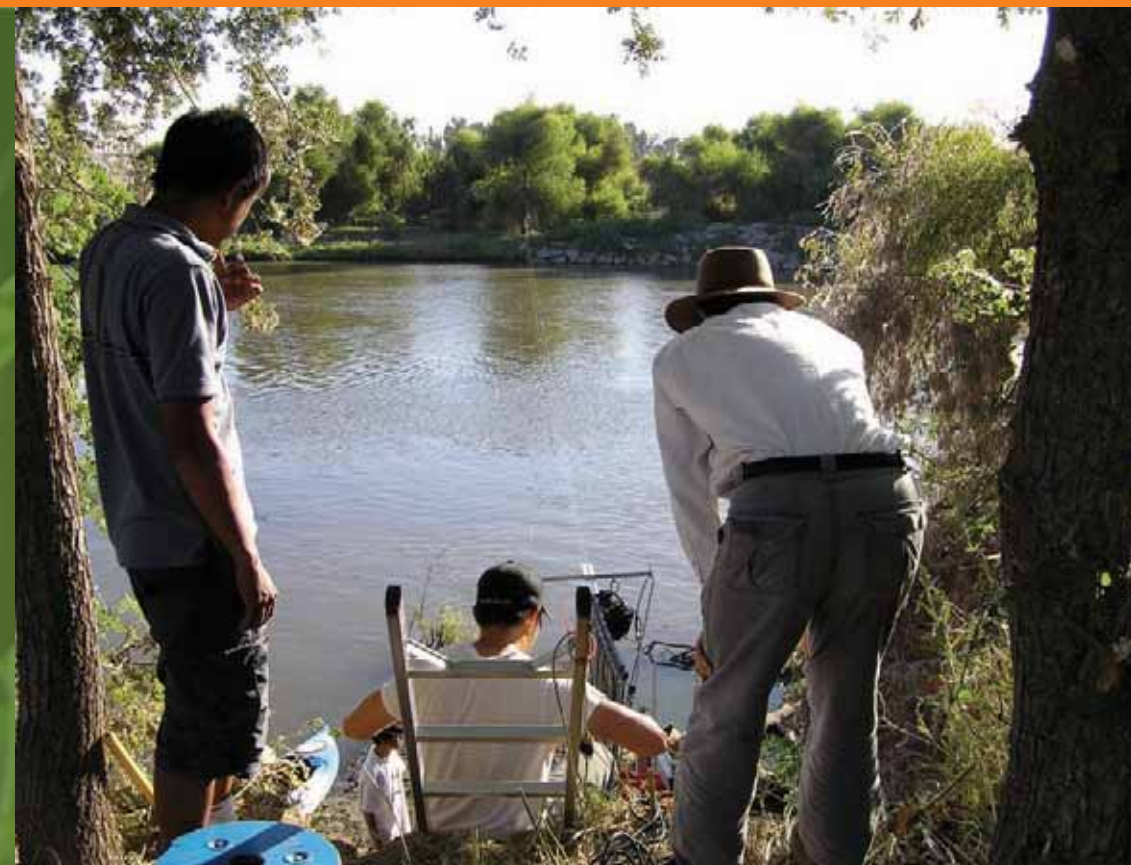
Engineers for CENS installing a robotic sensing system on the San Joaquin River in the California central valley.
