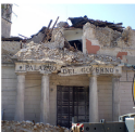
AF FAULT: A government building severely damaged by the April 2009 magnitude 6.3 earthquake in L'Aquila, Italy. Image Courtesy of TheItalySite via Wikimedia Commons
